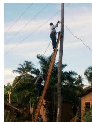
Electricity Reaches Lihami
